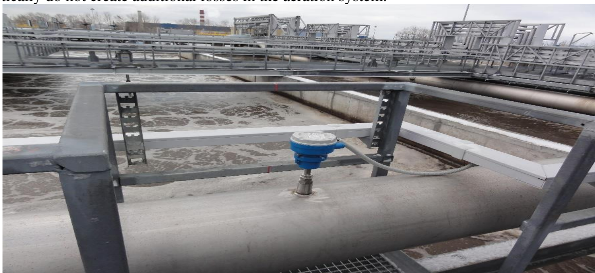
Fig.2. Thermal mass flow meter on the supply pipeline
