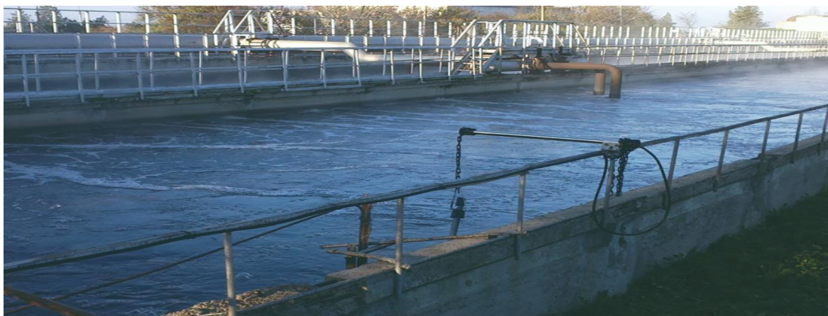
Fig.1. In-line dissolved oxygen sensor, installation on the side of an aeration tank
